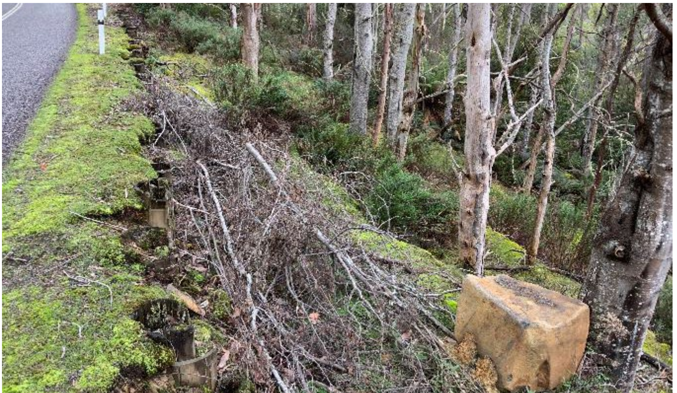
Photo 4: View looking northwest of 2009 remediated failure beneath Lyell Highway. Timber posts presumably installed as part of these works are heavily degraded. A distinctive benched profile is visible downslope. Note cubic rock block in foreground of photograph is associated with an isolated mechanism.
