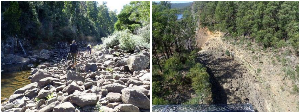
Figure 6.40: (left) River Derwent within 300 m downstream of Wayatinah Lagoon (right) eroding riverbank downstream of Wayatinah Dam.
