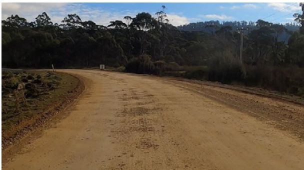
Figure 6: Butlers Gorge Road - evidence of minor corrugations (-42.266, 146.291)
