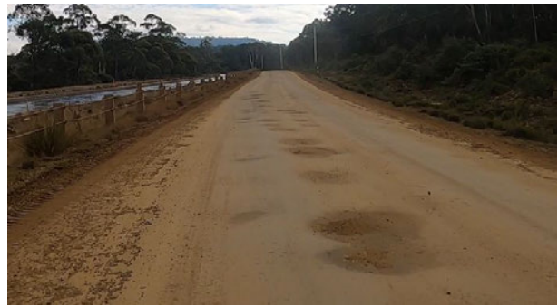
Figure 5: Butlers Gorge Road - evidence of minor potholes (-42.267, 146.316)
