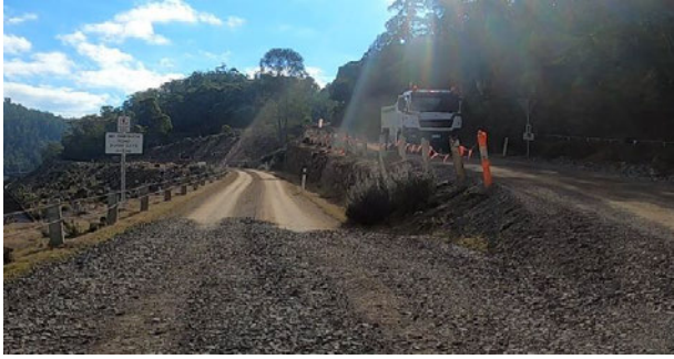
Figure 8: Butlers Gorge Road - road safety barrier (-42.273, 146.269)
