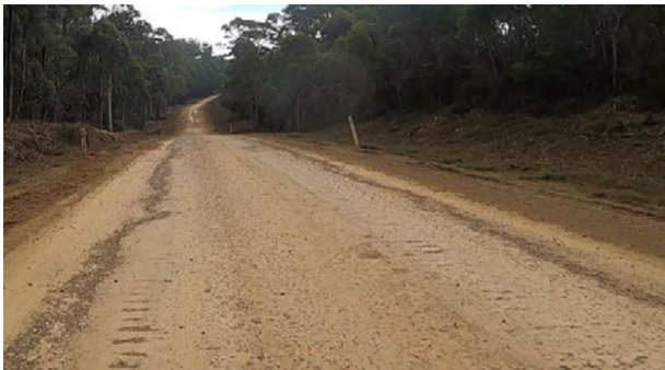
Figure 4: Butlers Gorge Road - evidence of longitudinal scouring (-42.282, 146.400)
