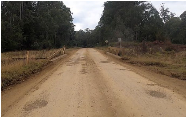
Figure 10: Fourteen Mile Road - evidence of minor potholes (-42.301, 146.422)
