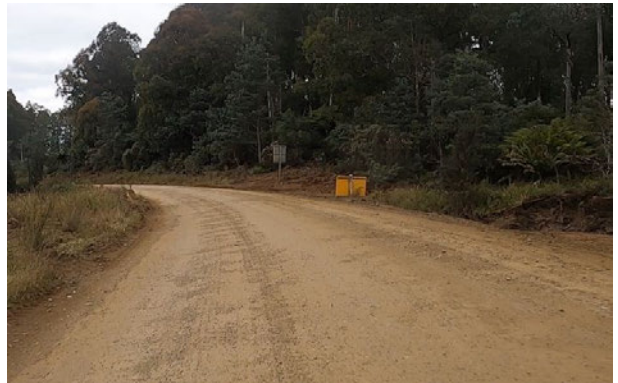
Figure 11: Fourteen Mile Road - evidence of minor corrugations (-42.304, 146.421)
