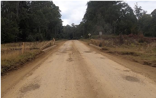
Figure 10: Fourteen Mile Road - evidence of minor potholes (-42.301, 146.422)
