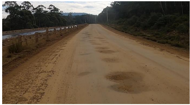
Figure 5: Butlers Gorge Road - evidence of minor potholes (-42.267, 146.316)
