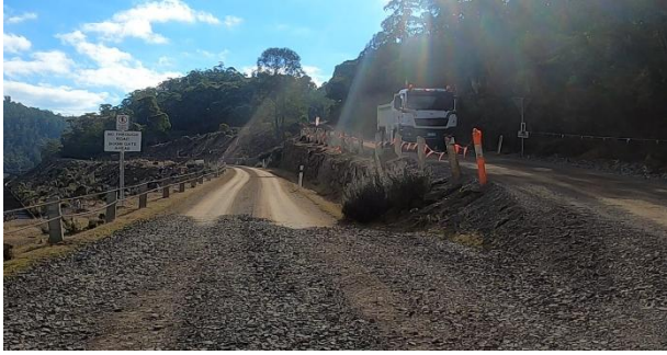
Figure 8: Butlers Gorge Road - road safety barrier (-42.273, 146.269)
