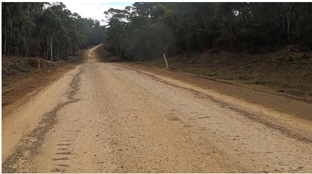
Figure 4: Butlers Gorge Road - evidence of longitudinal scouring (-42.282, 146.400)
