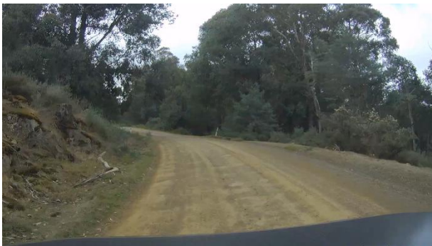
Figure 12: Victoria Valley Road - evidence of minor corrugations (-42.188, 146.511)
