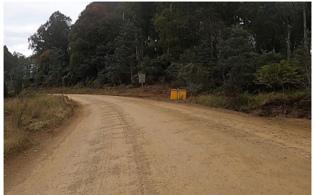
Figure 11: Fourteen Mile Road - evidence of minor corrugations (-42.304, 146.421)
