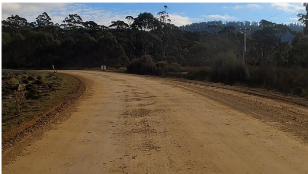
Figure 6: Butlers Gorge Road - evidence of minor corrugations (-42.266, 146.291)
