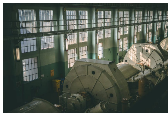
Figure 29: Turbines at Tarraleah Power Station
