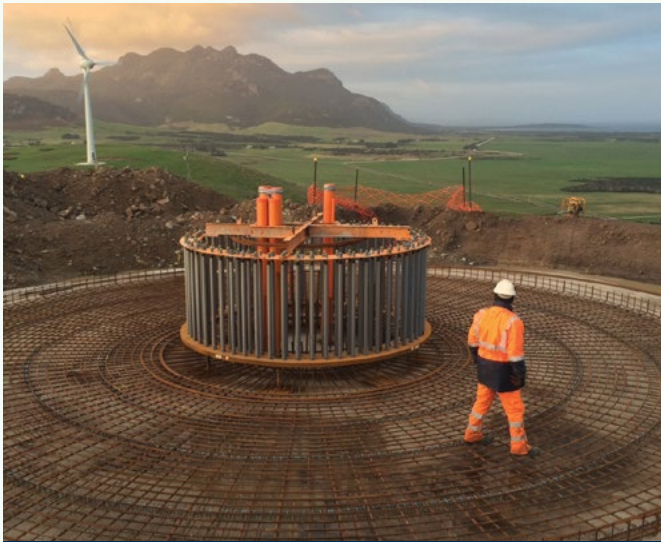
Wind turbine foundation
