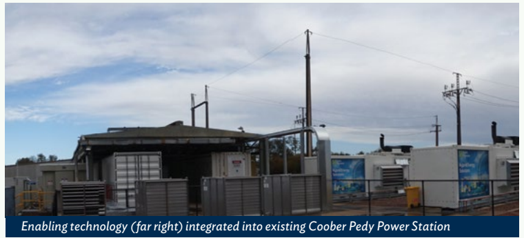
Enabling technology (far right) integrated into existing Cooper Pedy Power Station
