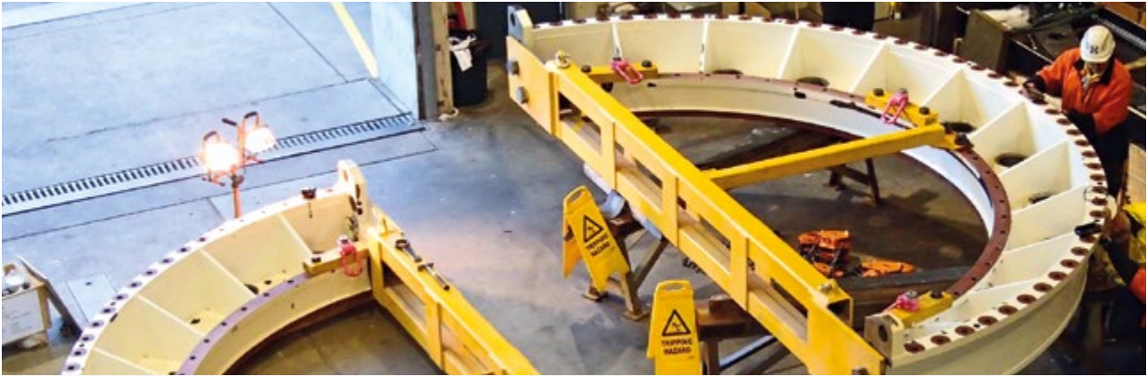
Refurbished outer top cover of a turbine during the upgrade of Paloona Power Station
