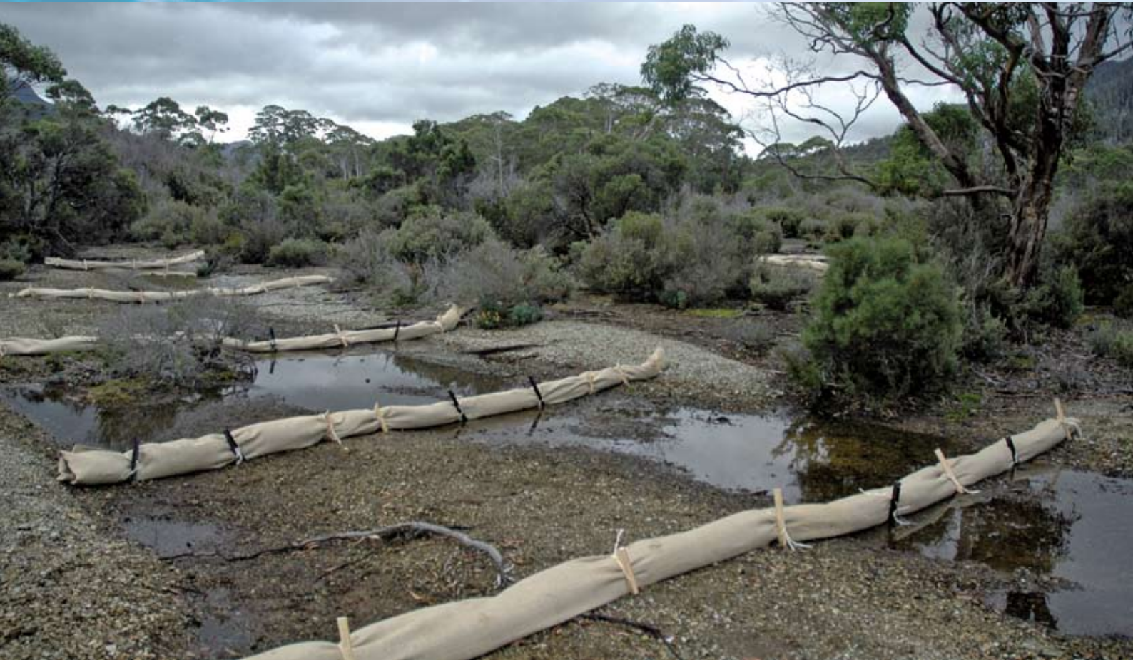
Hessian and jute rolls in place over an erosion-affected area at Narcissus
