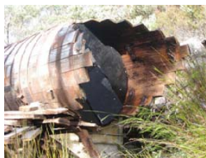
Woodstave pipeline and land slippage at Lake Margaret
