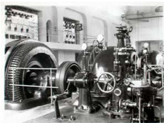
Original generator fit out, Lake Margaret power station
