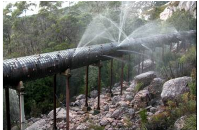
The wooden pipeline at Lake Margaret
