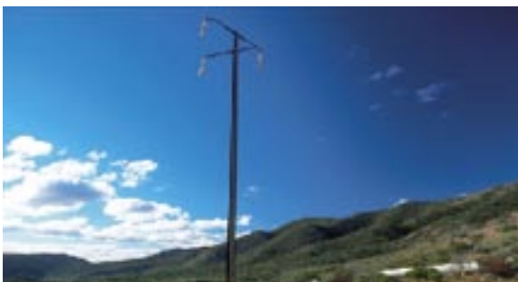
Example of Transmission tower, the Stobie pole
